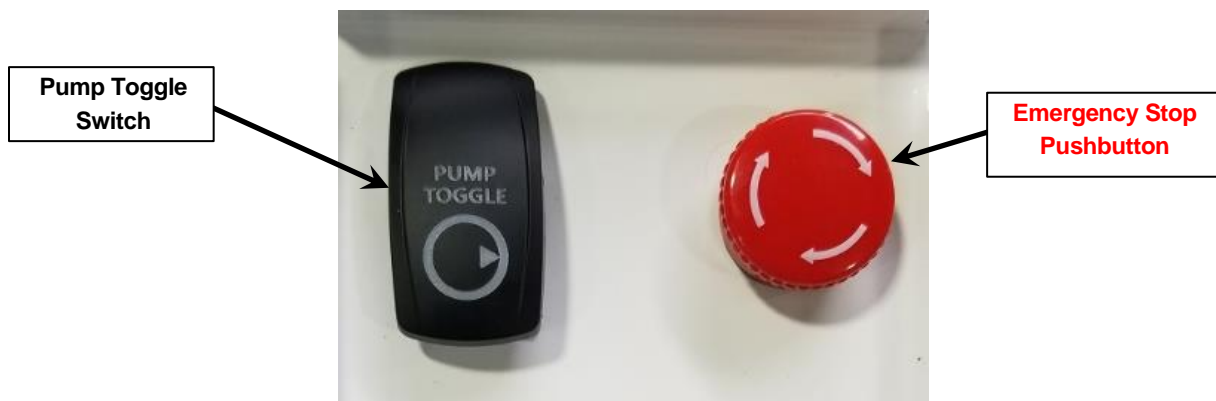
Figure 5. Pump Toggle Switch
