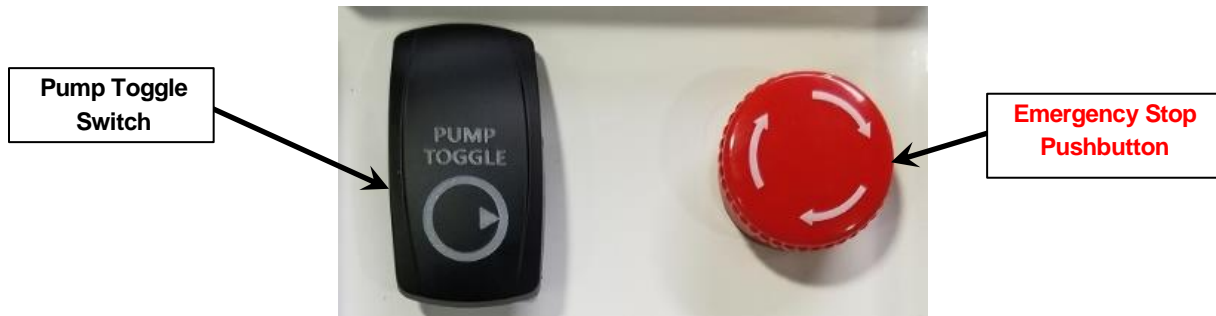
Figure 25. Pump Toggle Switch
