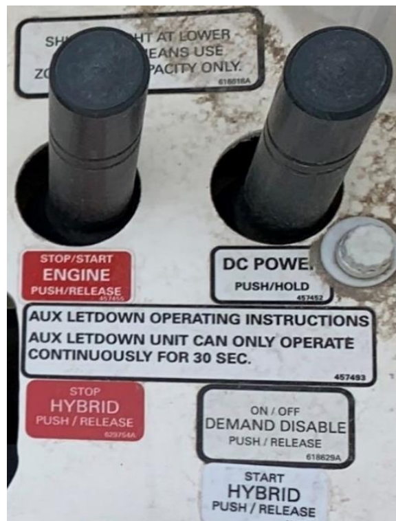
Figure 23. Typical Bucket Mounted Engine Start-Stop Controls
